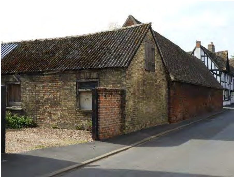
Gault and red brick barns adjoining a timber framed farmhouse, The Gables, Godmanchester
